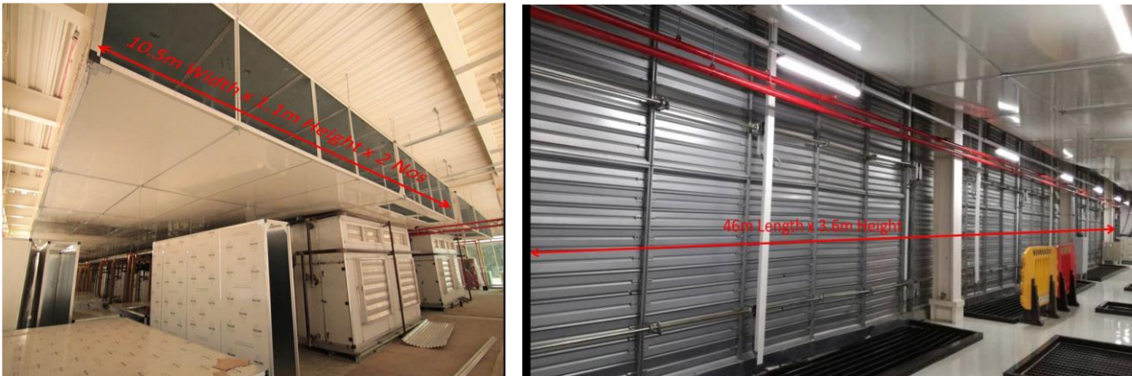
Figure 4. Fresh air intake and exhaust through motorized dampers. Both the intake and exhaust are directly above the server hall.
