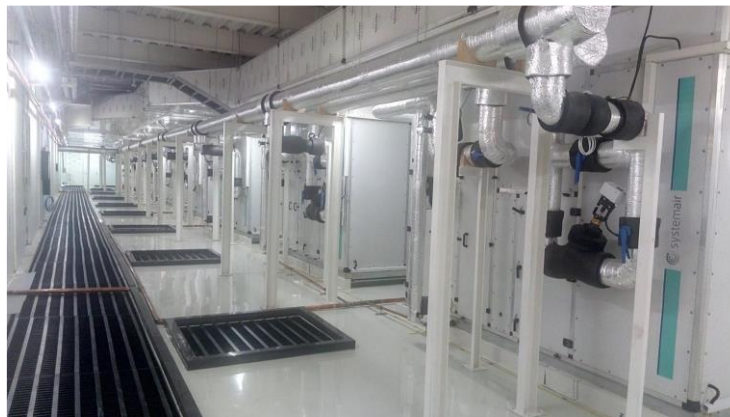
Figure 5. Air flows through vents next to the air-handling units, providing shorter air cycles and higher efficiency.
