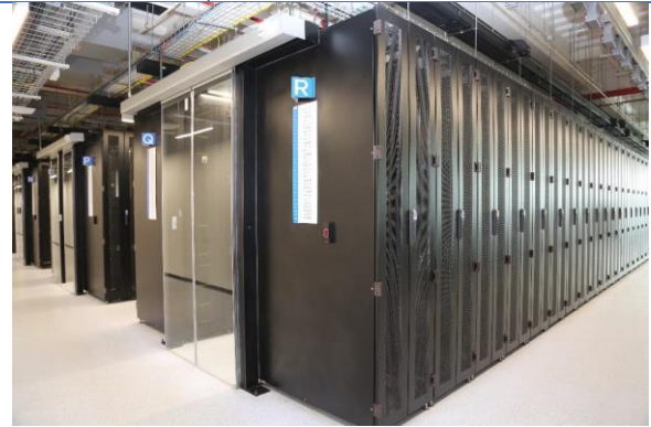
Figure 2. Data center server floor with air containment system
